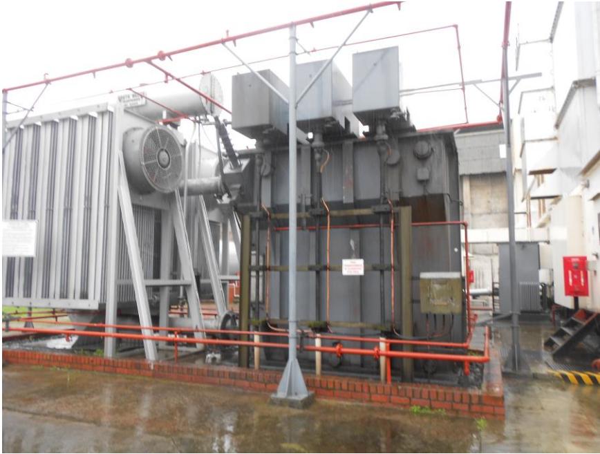
Figure 2: Back view of Athlone 11/66kV generator transformer.
