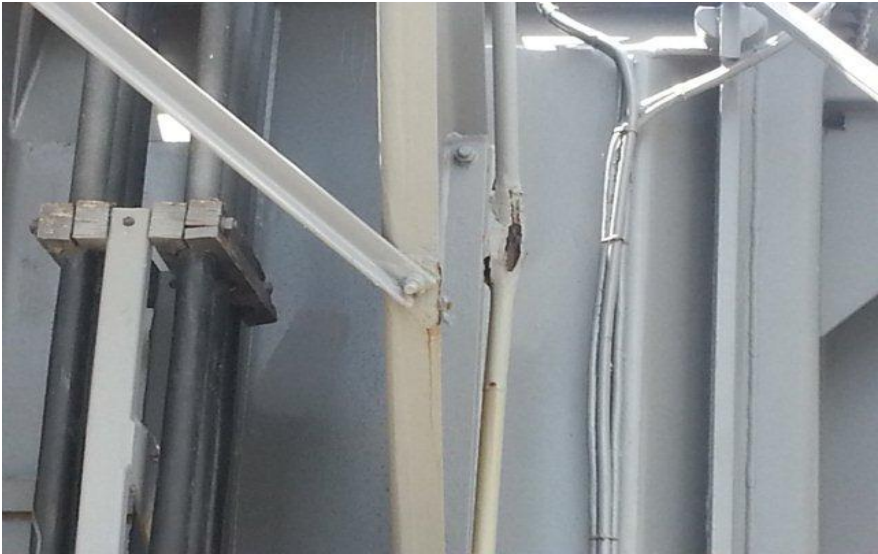
Figure 3: Mount Rd Gas turbine 11/66kV step up transformer
