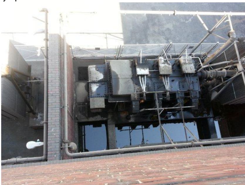
Figure 1: Top view of Pretoria West Power Station 11/132kV Generator step up transformer
